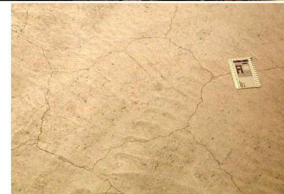
early age drying shrinkage cracks in a concrete pavement
