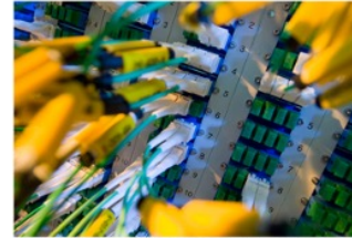
Grid Computing Centre Karlsruhe (GridKa)
