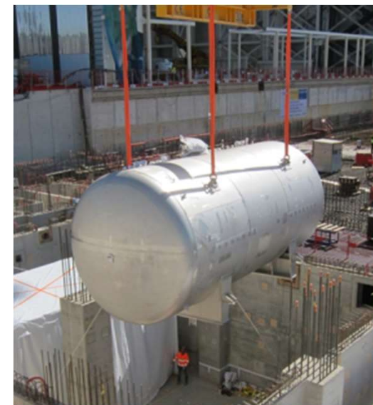
Emergency tank (100 m 3 )
