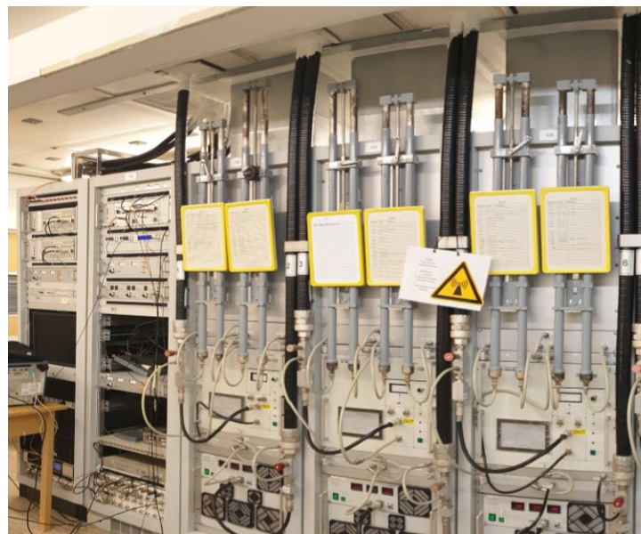
L-MBFB Rack, HPAs and phase shifters
