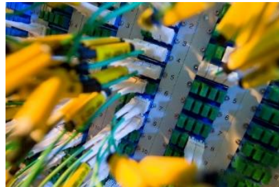
Grid Computing Centre Karlsruhe (GridKa)
