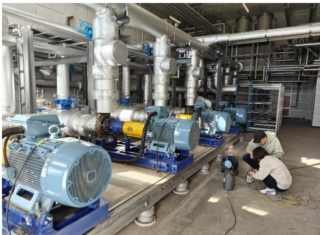
CW10 pump HIGH ENERGY PHOTON SOURCE
